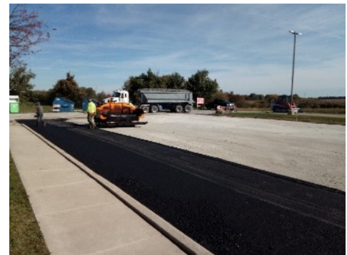
Workers begin laying asphalt on the Township Center parking lot on October 17
